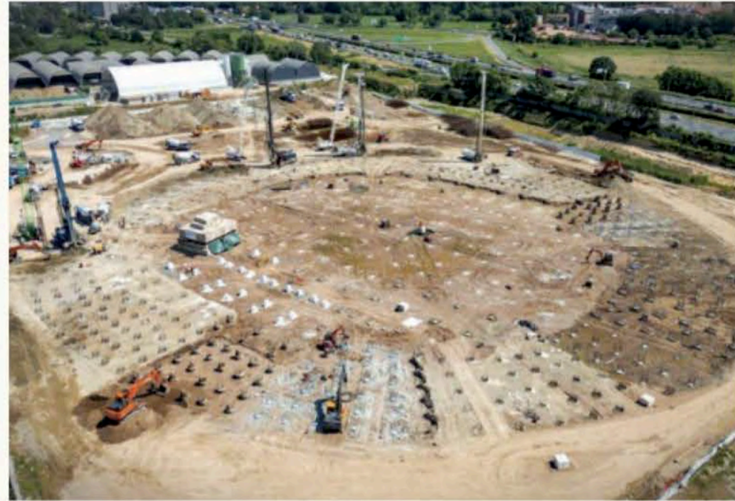
Trevi completed the foundation works for the new Santa Giulia Arena on schedule
