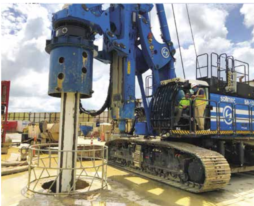
➤ A Soilmec SR-125 piling rig was used to drill into the embankment Picture: https://twitter.com/BooneRepair/status/1278710045535023107/photo/1
