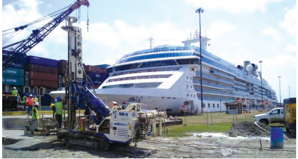
Soilmec SM-8 microdrilling rig drills and injects grout for the Borinquen Dam 1E foundation
