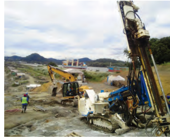
Drilling and grouting for Borinquen Dam 1E using a Soilmec SM-8 rig
