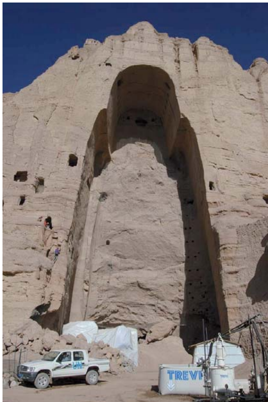
Permanent injection - Bamiyan, Afghanistan. Consolidation injections of the rocks of the niche of the Great Buddha.
