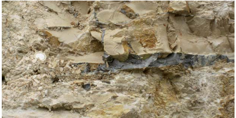
Cement grout injected in the joints of limestone formation (Bari, underground car park in Piazza Cesare Battisti, 2007).
