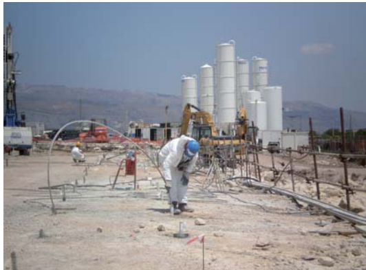
Manfredonia, Landfill of Conte di Troia (2010) Waterproofing injections in rock formation: MPSP installation and grouting
