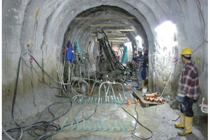
Temporary injection - Naples Underground, Toledo station. Pre-consolidation and waterproofing injections of the service tunnel.
