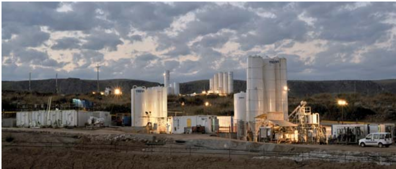
Grout preparation plants
